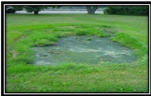
Failed Septic System
