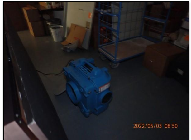
Figure (10) – Air scrubber located in Room 4.
