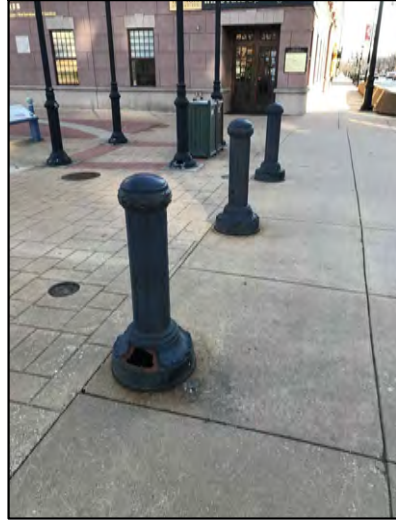
Replace damaged bollards/light poles
