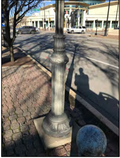
Paint faded/peeling light poles
