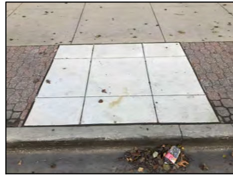
Previous tree location with concrete patch
