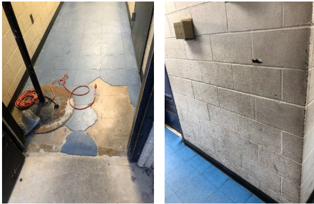
Figure 3: Before DPW improvements July 2024
