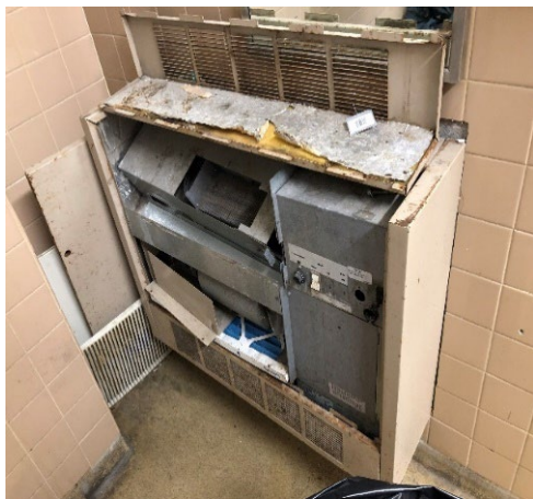
Figure 5: Before DPW improvements July 2024
