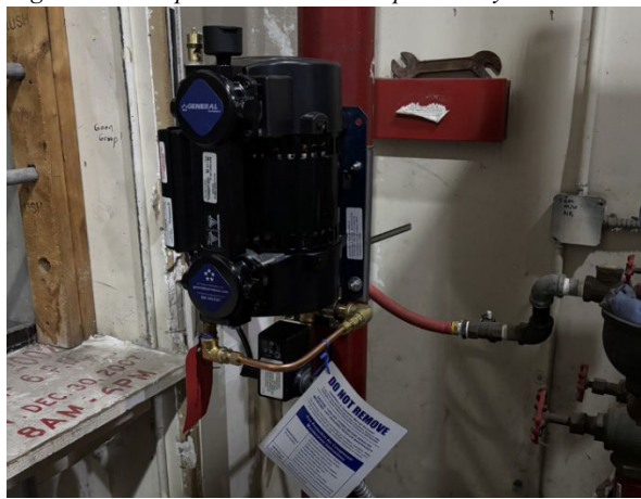
Figure 12: Compressor attached to sprinkler system
