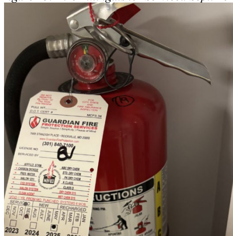
Figure 13: Fire Extinguisher Serviced Sept. 2025
