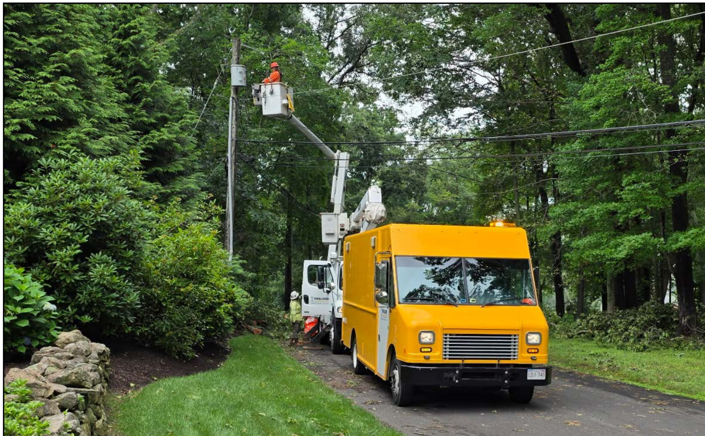
Crews work to restore power in New Canaan as Rep. Tom O’Dea and Sen. Ryan Fazio were out surveying the damage. Photo contributed by Tom O’Dea.
